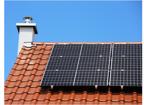
Figure 2 – Solar PV systems on new low-rise residential buildings is a new 2019 Energy Code requirement
